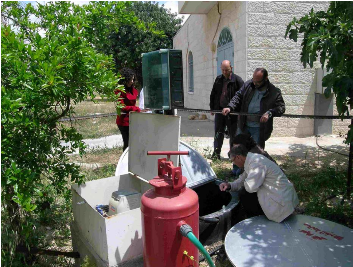
Photo 4. The full system. In the foreground we see the sand filter. The open tank is the micro water treatment plant. On top is the control and programming unit. The closed tank stores the treated water. The compressor is in the white box behind the sand filter.
