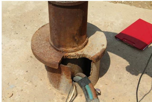
Figure 31: Open cable installation at the well head
