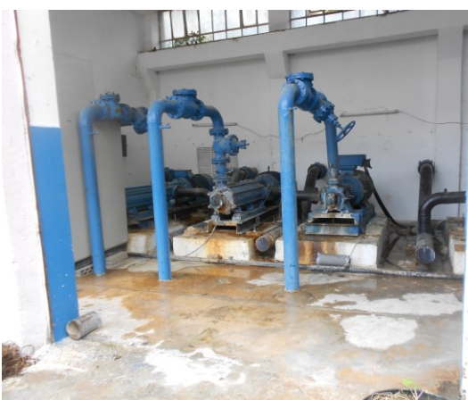
Figure 15: Yesidia wells pumping station (Zemann, 2012)
