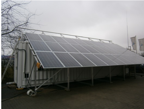
Figure 6: Container-based water treatment plant with solar plant (photo: SPA).
