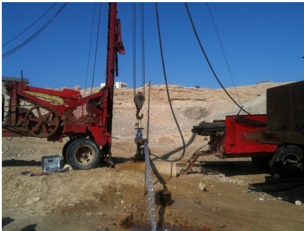
Figure 3: Pump experiments, Karameh well, Jordan (photo: MWI).
