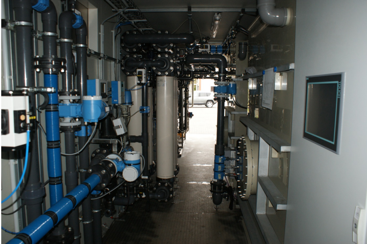
Figure 5: Water treatment plant (test run in Bremen, photo: SPA).
