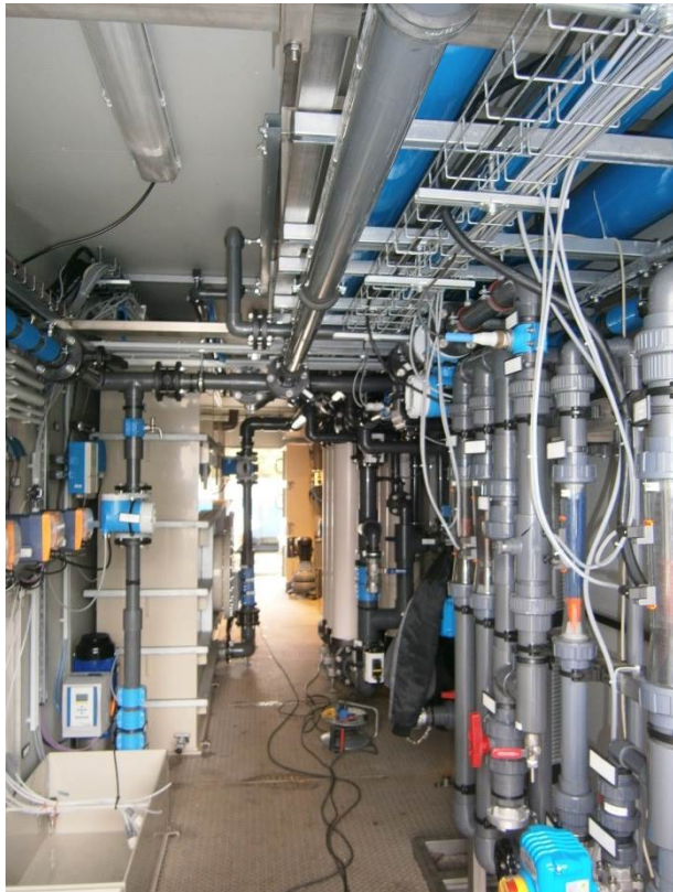
Figure 8: A view into the container. The reverse osmosis unit can be seen in the right-hand place in front, the ultrafiltration modules behind it. In the back is the aerator. Left hand, the dosing stations for chemicals and the backwash tanks are placed (photo: SPA).
