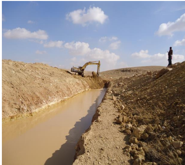
Pic. 13: Excavations showing rain filled the trench of the trench
