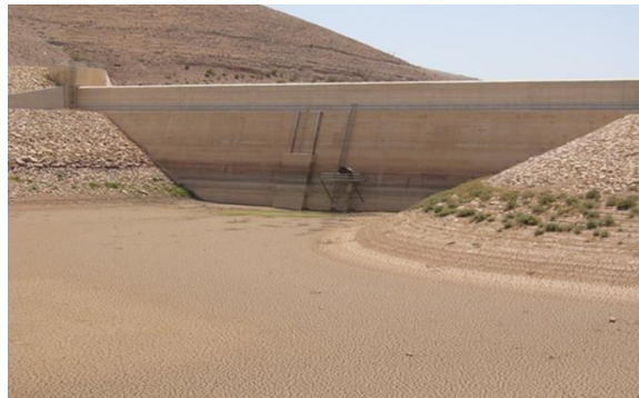
Figure 5: Wala Reservoir, August 2008.
