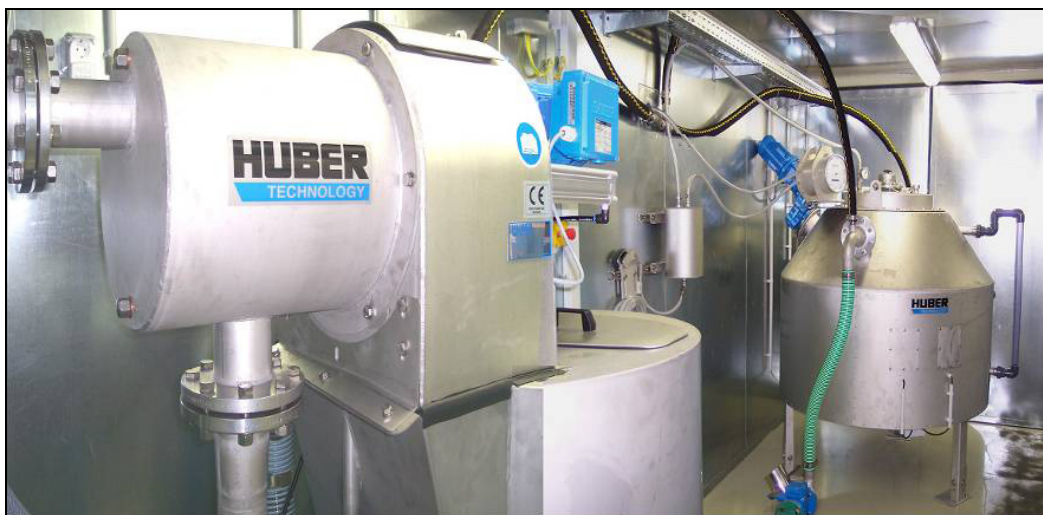
Figure 7: Anaerobic bioreactor plant at Fuhais (inside view)
