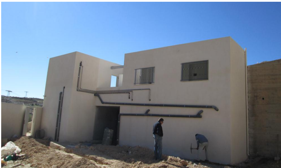
Figure 7: Backside of building with pipes
