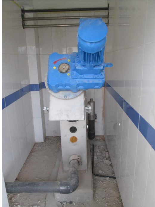
Figure 3: Ro9E fine screen during installation in separate screen room on Maghareeb site
