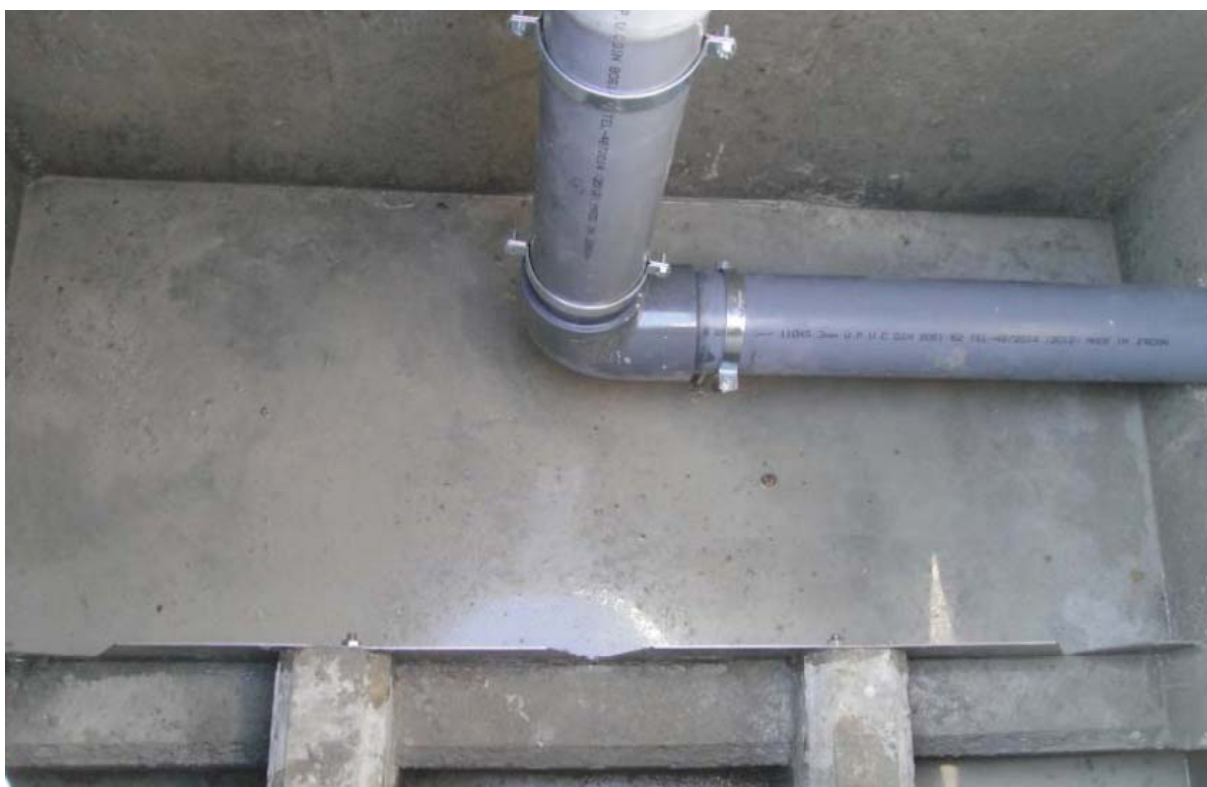
Figure 38: Interior of the flow splitting box.
